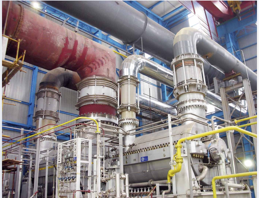
Compressor train at Wuhan plant
